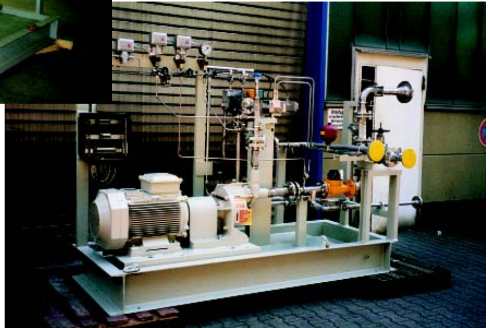
Pumping Stations for Oil Firing Installations and Injection Water
